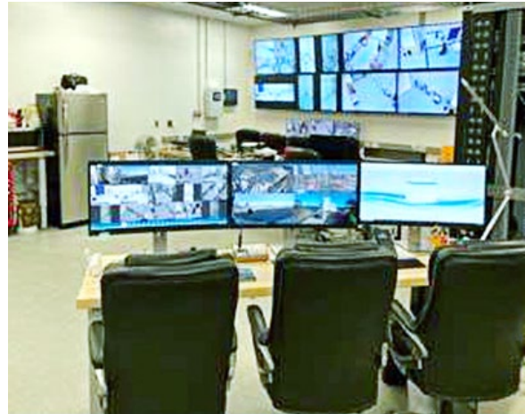
Figure 88: MARS Payload Processing Facility Control Systems
