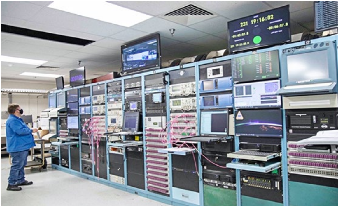
Figure 17: Telemetry Ground Station
